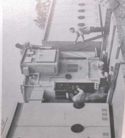
Work crew inspects trim and tidy Maekiki Substation, one of several such units located throughout city.
