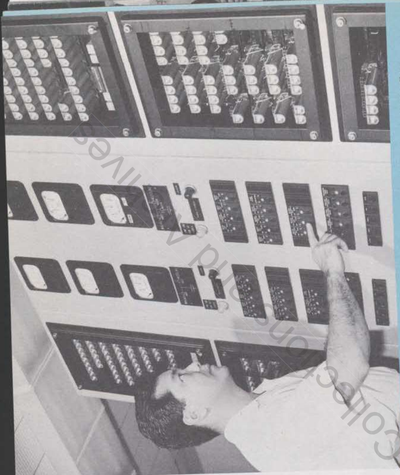
New electronic equipment speeds operations in load dispatcher's office, providing efficient remote controls for switching gear, meter reading.
