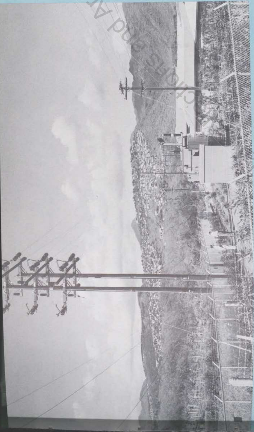
Expanding need for electric power in Waialae-Kahala district required new substation nearby. Cost of land, equipment and installation was $98,000.
