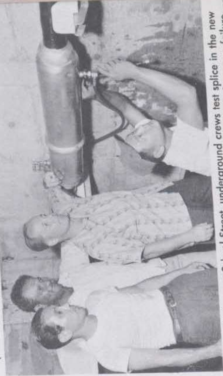
Gas-filled cable, the first used in the Territory, was installed to transmit power from new generating plant to Iwilei and School Street substations.
