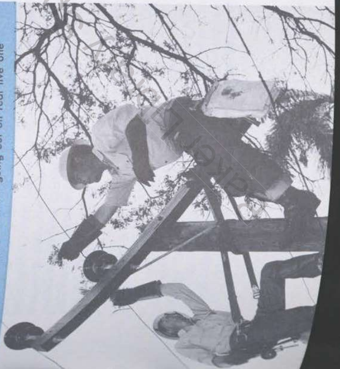
Carefully chosen apprentices learn lines instead of ropes. Teacher and pupil here work on dummy pole before going out on real live one
