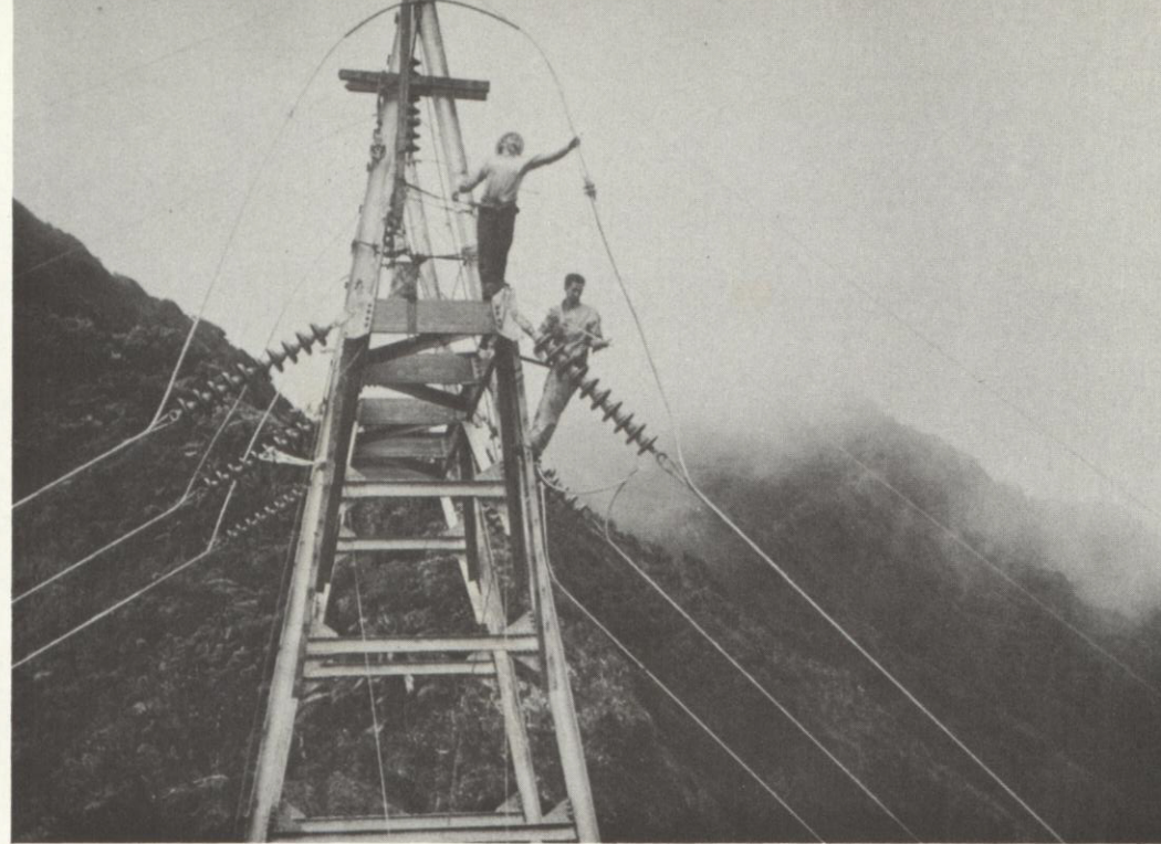
One of 50-foot aluminum towers atop Koolau range carrying new lines to transmit ultimately at 138 kv, serving Windward and Leeward Oahu.
