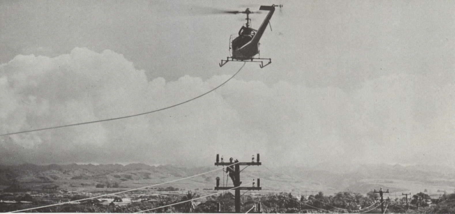
Helicopter is "sky hook" for stringing lines. By this method, 1 mile can be set in place in 10 minutes.
