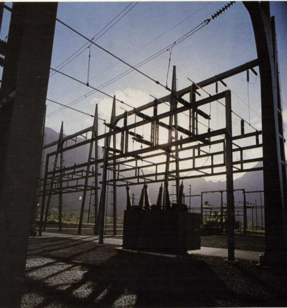
The Koolau Substation in late afternoon, as the sun settles behind the rugged Koolau Range.
