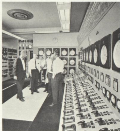
Nerve center of plant is the Control Room, serving both Kahe 1 and Kahe 2. The two plants are the company's 15th and 16th power-producing units.
