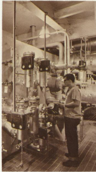
Water for the boiler must be purified. It is turned into steam in a flash evaporator, filtered, recondensed.
