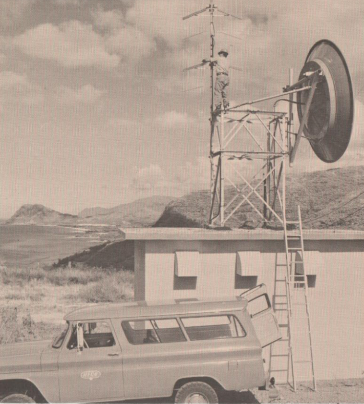
A modern microwave and mobile radio system, developed to monitor and control power plants and substations and to communicate with service crews, covers the Island.
