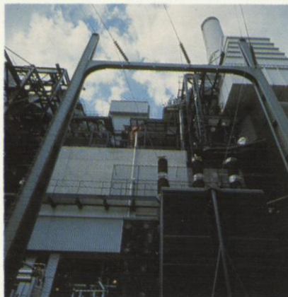
Kahe plants are outdoor type with boiler structure left unenclosed, saving building costs. Plant is most economical in system.
