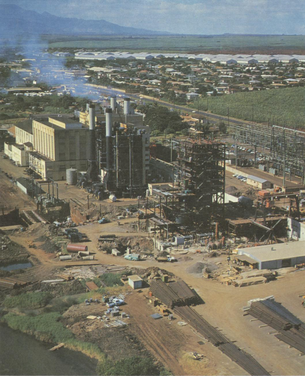
Waiiau Generating Station was center of expansion. Seventh unit under construction there at cost of $12.2 million will add 86,000 kilowatts to system when completed in late 1966.
