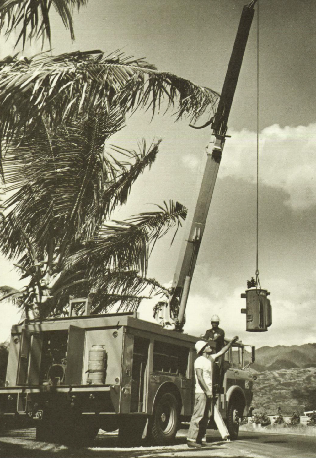
Low-silhouette line truck designed by Engineering Department was put into successful operation. Body is only 6 feet high. Tools and materials are easy to store and reach. Working foreman George Garcia, at controls, and James Smith, helper, demonstrate use of center-mount boom, clearly visible to operator over low roof.
