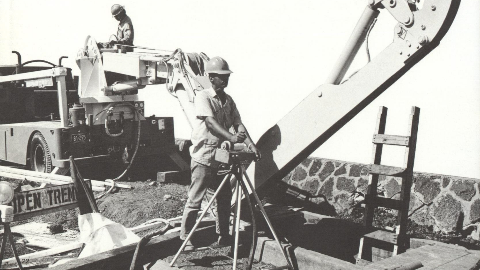
Efficient cable-puller is one of modern methods Company uses to extend underground wiring system
