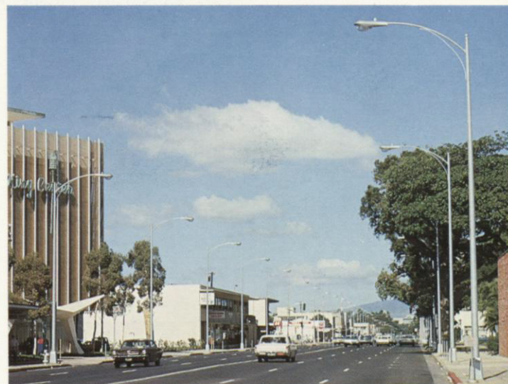
Street widening and undergrounding greatly improved appearance and traffic flow on a midtown section of King Street, Honolulu. Photos, top to bottom, show project before, during and after removal of lines and poles by Hawaiian Electric.
