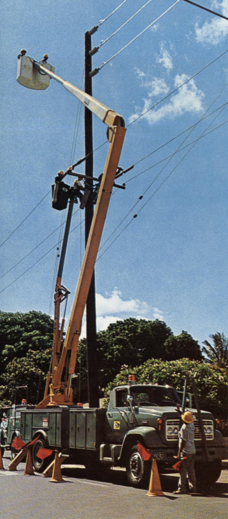
Linemen work comfortably and effectively at heights up to 70 feet in new Hi-Ranger bucket truck added to Company fleet.
