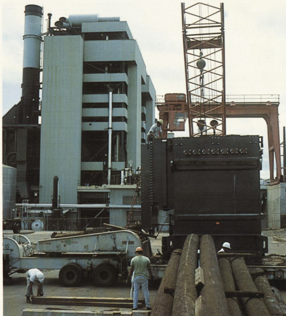
Transmission facilities increased in keeping with growing power demand on Oahu. New equipment in 1969 included transformer of 80-plus tons, shown being unloaded at Waiau Generating Station.
