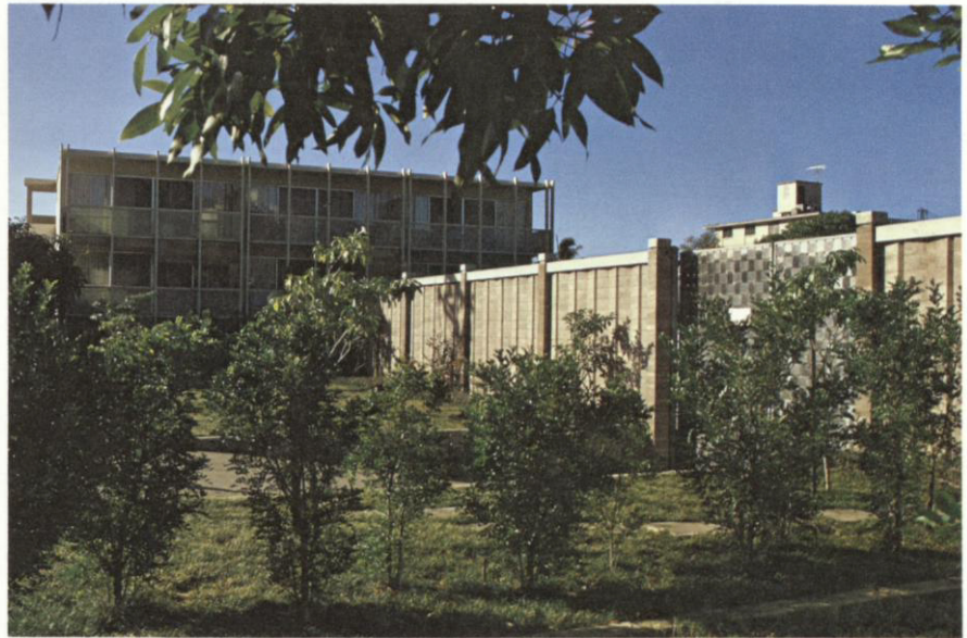
Decorative wall and doors, abundant planting and a low silhouette make this neighborhood substation inconspicuous, all part of Company beautification program.
