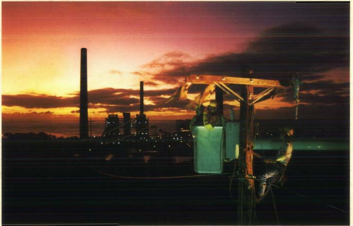
Framed by the silhouette of the Kahe power plant on Oahu, HECO linemen (left to right) Stephen Keith, Jason Sampang and Neil Munemitsu work on a transformer during a training exercise at sunset.
