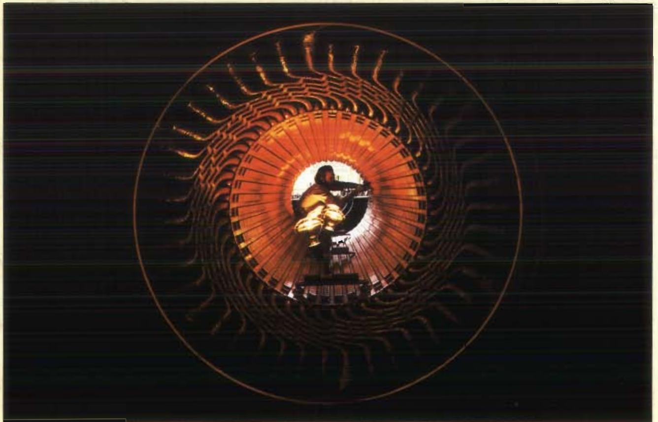
A generator armature, part of a 55-megawatt power unit at HECO's Waiau plant west of Honolulu, glows with special lighting as electrician Randy Whittington inspects the coils during routine maintenance.
