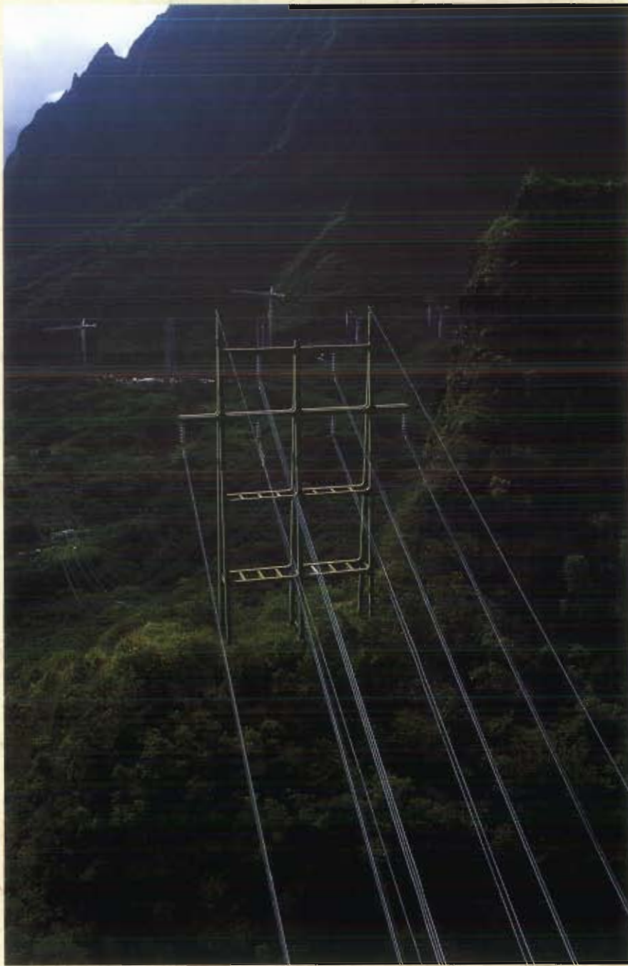
Massive 138-kilovolt transmission lines glisten in the morning sun along the windward ridges of Oahu's Koolau Mountains near Kaneohe.
