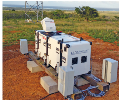
Hawaiian Electric has deployed a scanning "light detection and ranging" device at one of its O'ahu substations to forecast wind conditions in the area, allowing system operators to better adjust generator outputs to maintain reliable service.
