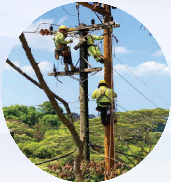
A Hawaiian Electric crew replaces utility poles that support the circuit feeding the Pacific Palisades neighborhood on Oahu. Replacing aging and damaged poles with stronger ones is one of the equipment upgrades we make to improve grid resilience and service reliability for our customers.
