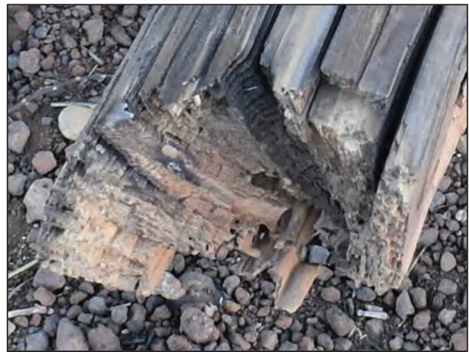
Figure 46: August 13, 2023 field photograph of the bottom Pole 7A fracture surface with the bored through-bolt hole visible
