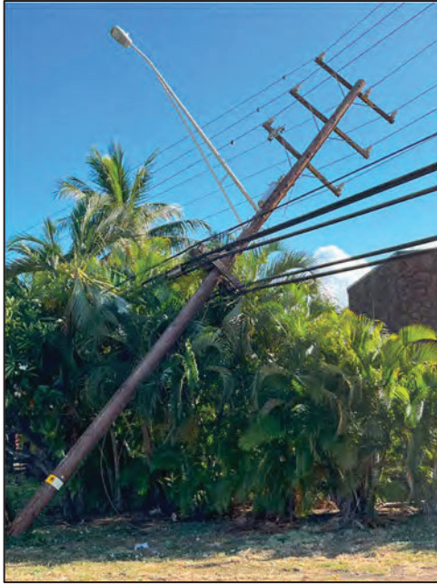
Figure 16: 8:00 a.m. photo captured by Hawaiian Electric foreman of Pole 13 leaning at the intersection of Honoapiilani Highway and Keawe Street
