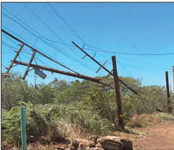
Figure 40: Photo captured by a Hawaiian Electric foreman at 2:27 p.m. of damaged poles and lines on Mill Street
