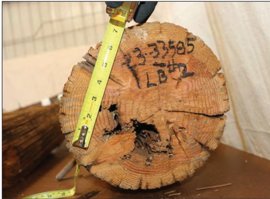
Figure 47: Photo captured February 2024. The photo presents a cross-section of Pole 7A above its fracture point. The photographed cut was made shortly after the August 8 fires when Pole 7A was removed from the field. An enclosed pocket, of mild to moderate termite damage is visible in the bottom left quadrant of the pole. Because the outer shell of Pole 7A is fully intact, the bulk of the pole's strength remained.
