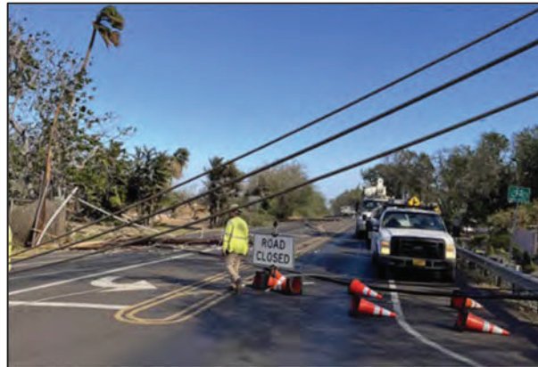
Figure 34: 4:33 p.m. south-facing photo captured by a Hawaiian Electric contractor showing additional poles and power lines down, as well as low-hanging telecommunications lines at Aholo Road fully blocking Honoapiilani Highway
