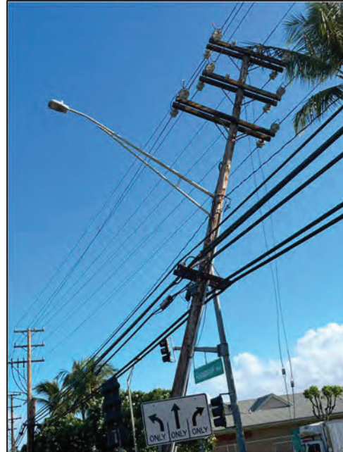
Figure 17: 8:01 a.m. photo captured by Hawaiian Electric foreman of Pole 14 leaning at the intersection of Honoapiilani Highway and Keawe Street
