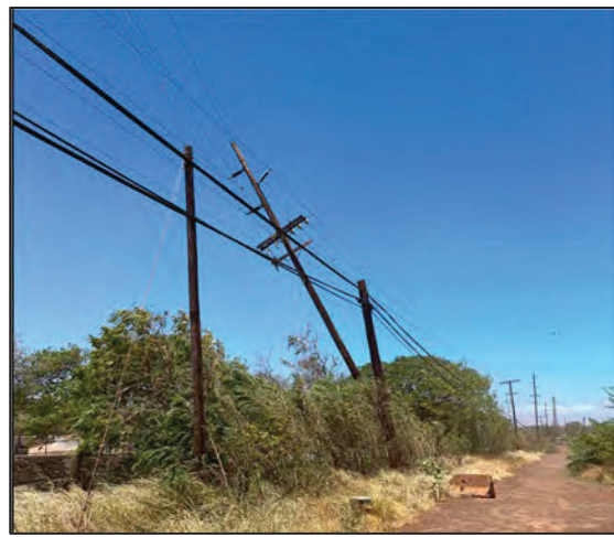
Figure 41: Photo captured by a Hawaiian Electric foreman at 12:37 p.m. of damaged poles and lines on Mill Street
