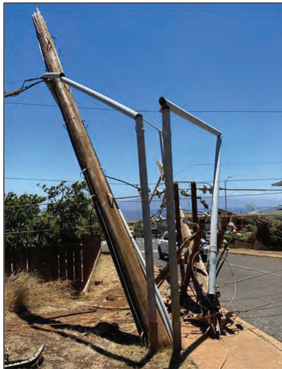
Figure 23: 1:21 p.m. photo captured by a Hawaiian Electric foreman of Pole 8 at Kumukahi Street and Ho'okahua Street leaning toward the backyard of a residence
