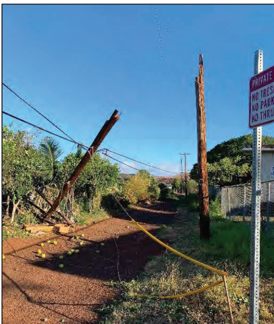
Figure 13: 7:29 a.m. photo captured by a Hawaiian Electric Troublemán showing Pole 7A snapped in half. The base of Pole 7A remains upright and in the ground
